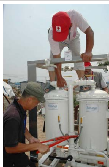
RCSC team members operate the M15 water ERU independently, after having been trained in all aspects of ERU operations and maintenance by the Austrian Red Cross. Photo: Mike Wolf/International Federation.
