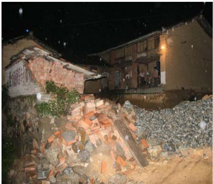
A house in Renhe district of Panzhihua city, damaged in the earthquake measuring 6.1 on the Richter (Photo: Xinhua)
