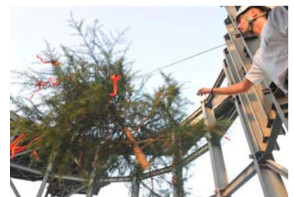
A tree is raised to the roof of the Swiss Pavilion, following the same path that visitors to the Pavilion will take as they ride the chair lift from the ground floor to the pavilion roof – a journey that is meant to symbolize the interconnection between urban and rural spaces.
