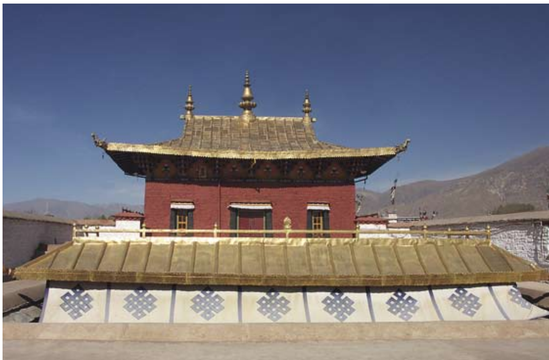
(Fig. 2) View of the roof of Ramoche showing completed restoration work (Photography by Mi Nyag Rinpoche Chökyi Gyaltzen)
